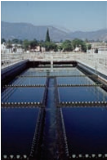
Water undergoes optimized conventional pretreatment prior to reverse osmosis.
